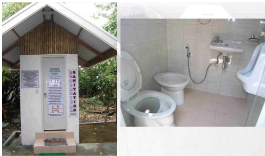
Figure 3. Ecological sanitation toilet in an urban setting. Courtesy of the center for advance Philippine studies.
