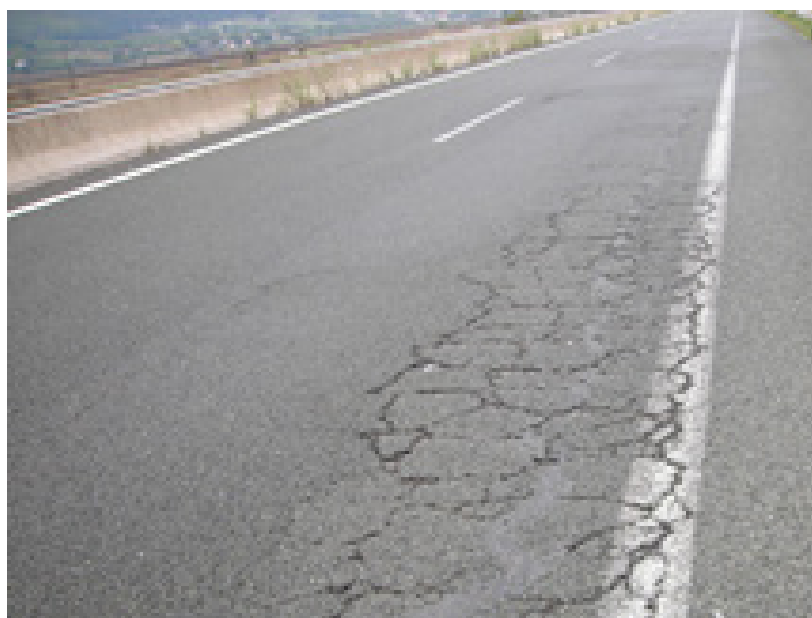
Figure 1. Poor road serviceability due to surface cracks: Urgent need for maintenance on toll motorway.
