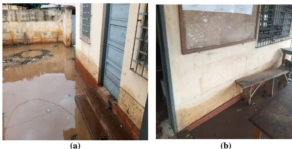
Figure 2. Flooded health facilities. (a) in front of the medical consultation room; (b) in front of the Sanitation-Vaccination department.
