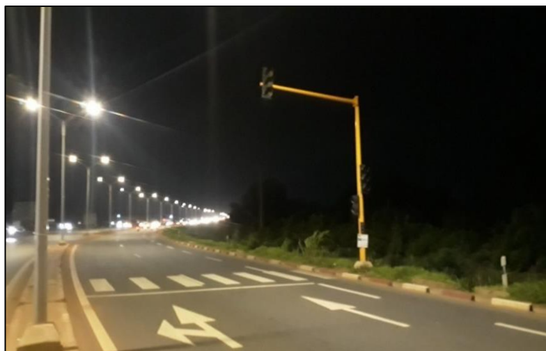
Figure 3. Malfunctioning traffic light on ECOWAS Boulevard.
