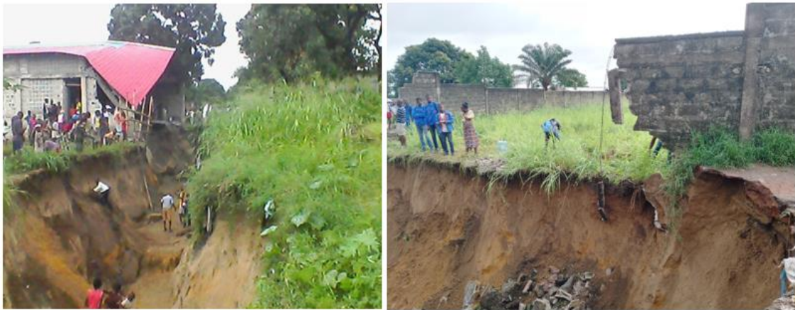
Figure 11. Destruction of dwelling by erosion.
